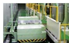
Harima Plant: New Microelectronics Production Facility (internal equipment)
